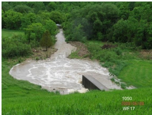
West Fork 17 Stilling Basin Damage – June 2008
